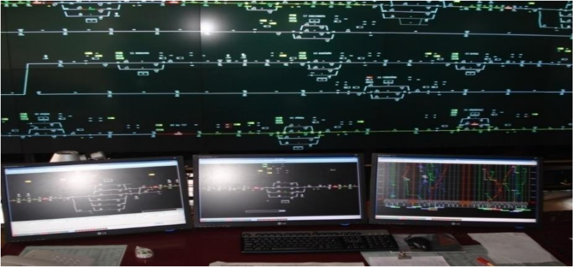
Figure 4: Traffic Control Panel
