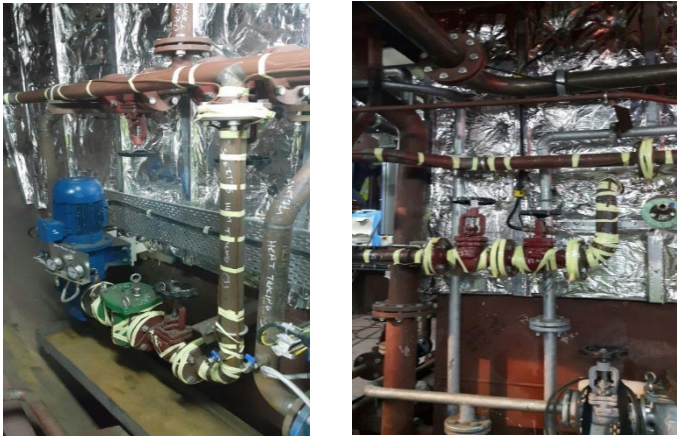
Fig. 1 Application of an electrical heat tracing system on board.
